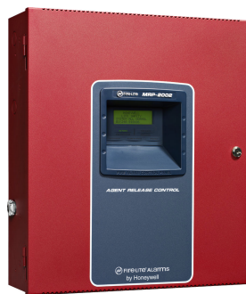
Fire control panel
